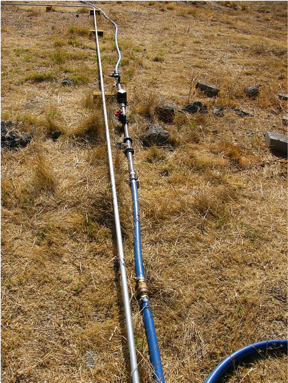
Pipe Connection and Valves from GW-16
